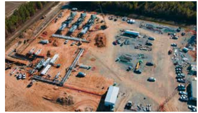
Chesapeake: North Louisiana Natural Gas Treating Facility.
